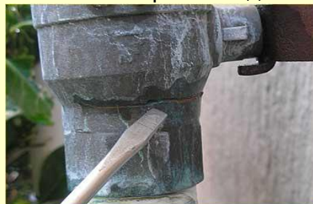
Frozen Pipes Cost $$
